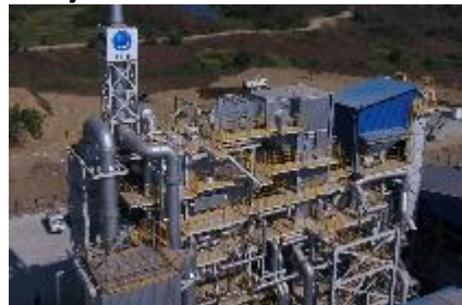
【Waste to Energy plant】 (Myanmar) 4,732tCO 2 /y. Start operation: Apr. 2017
