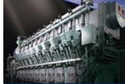
【Co-Generation Plant】 (Thailand) 7,308tCO 2 /y. Start operation Apr. 2018
